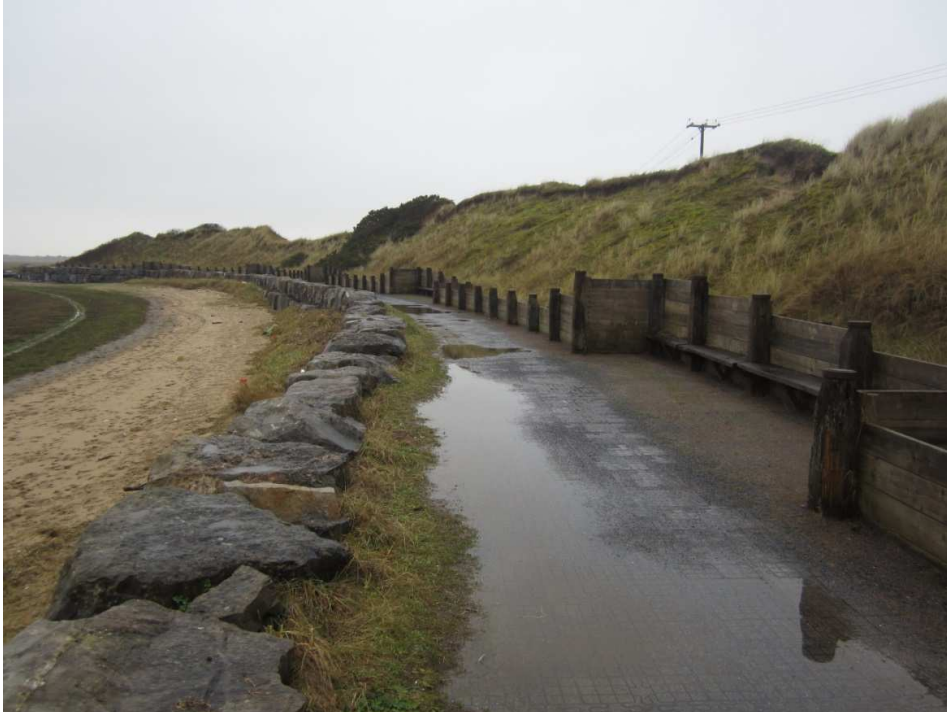
Photograph 25: Coast protection works and stabilized dunes to the west of Pembrey Old Harbour.
