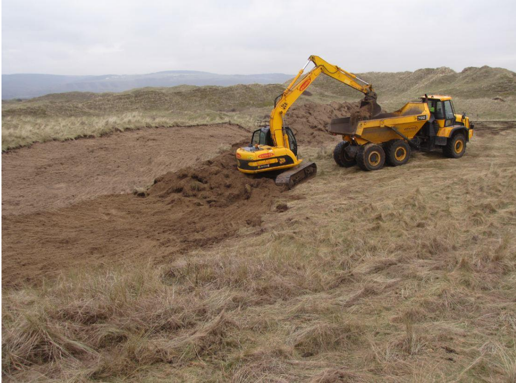
Figure 2. Turf stripping, Kenfig Phase 1, February 2012 (photograph supplied by David Carrington, Bridgend Borough Council).
